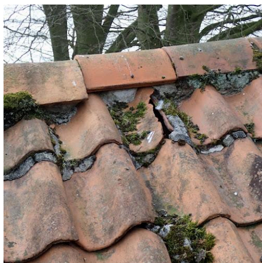
dak [1]-noord: gebroken pan
