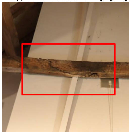
zolder [2]-noord: gebroken trek balk
