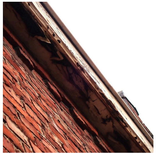
dak [1]-zuid: ingerotte gootbekleding
