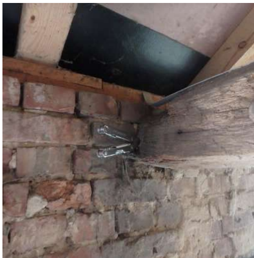
zolder [5]: ingerotte moerbalk
