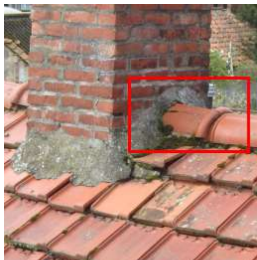
dak [2]: gebroken nokpan
